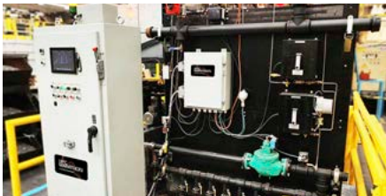
Gas generator for fastener manufacturer
