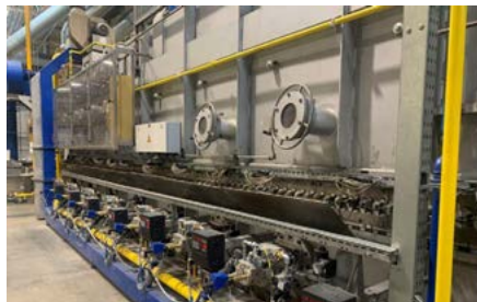
Indirectly heated roller hearth furnace
