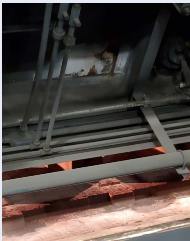
Heat-damaged case wall
