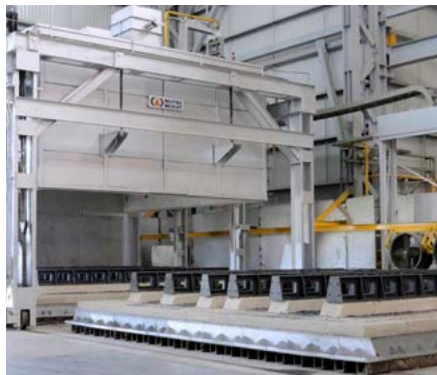
One of five lift-up furnaces for closed-die forgings
