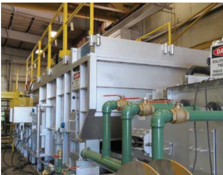
Continuous quench and temper furnace system for a North American producer
