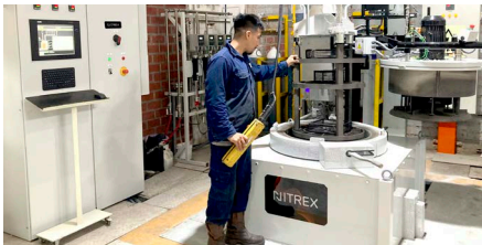
New pit-type furnace for voestalpine High Performance Metals del Perú
