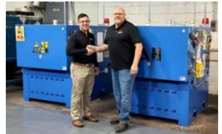
Twin convection furnaces for tempering
