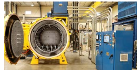
Firearms manufacturer with in-house heat treating
